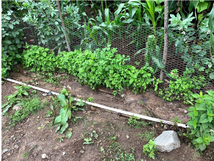
Photo 1: Existing water distribution system exposed near the main road running through the community.
