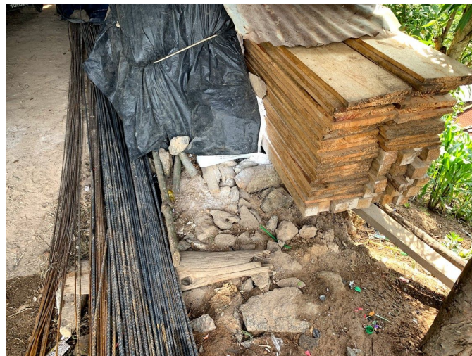
Photo 6: Rebar and wood framing used in the construction of a new house in the community.
