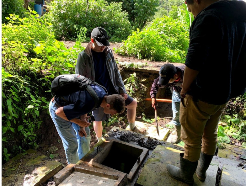
Photo 3: Members of COCODE and EWB-KC evaluating the structure that divides water flow from the source between Los Churuneles II and two other nearby communities.
